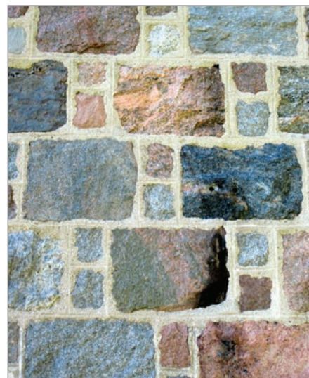
FIG. 17. CRELLIN'S ABERDEEN BOND STYLE MASONRY WITH 2 SNECKS, MCCOMB HOUSE, 1 33 RD LINE, NO. 6603, NEAR HARRINGTON, OXFORD COUNTY. | KAREN E. ARMSTRONG.
