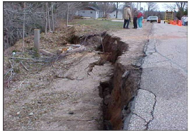
Figure 10. A large rotational slump in Middleton, Nova Scotia. This landslide was associated with fluvial erosion of 20 m-high slope along the Annapolis River when the water table was elevated activating a failure plane between impermeable clay-rich till and overlying outwash sediment.
