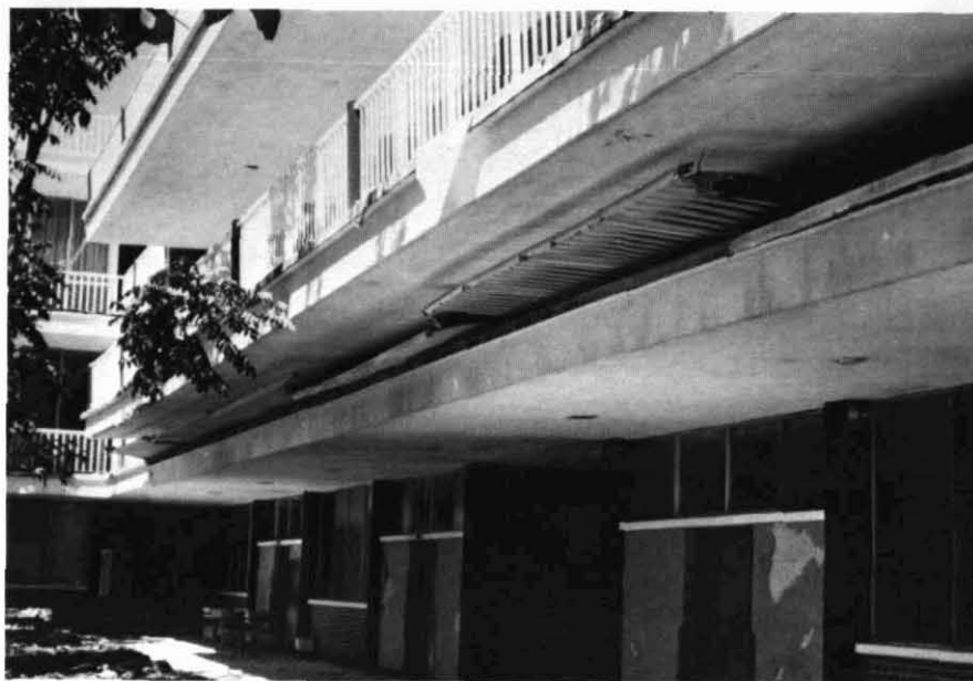
Figure 7 Collapsed second floor of a school in southeast Guatemala City, about 30 km from fault.
