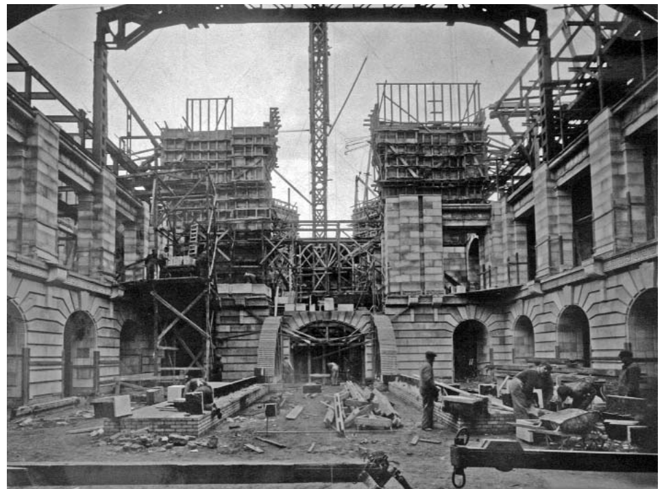
Figure 3. 1916; the grand staircase area on the main floor (AM, Foote Collection 78). Workers lay brick and steel supports to prepare the base of the grand staircase for its railings, addition of the Tyndall Stone facing and placement of the two bronze bison that flank the staircase ( see Figure 8a).
