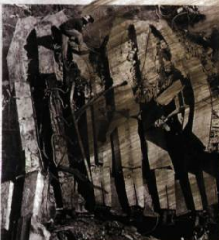
The Remains of a Tower A worker beamed himself against the rubble as he broke apart what is left of the facade of 1 World Trade Center yesterday. Many people still say the search and that some ground zero make the area unpleasant.
