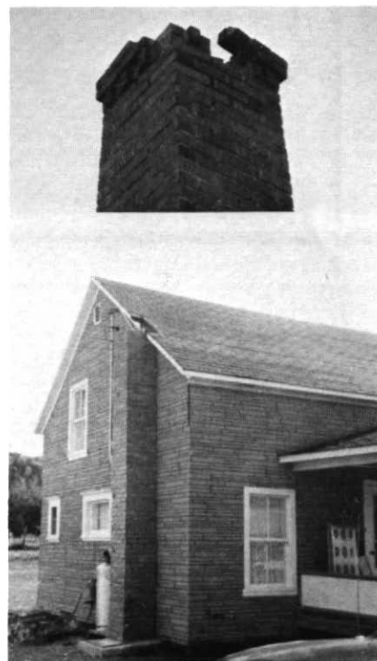
Figure 4 June 14, 1973. Chimney damage at Woburn, Québec. Most chimneys in the town were undamaged. (Fig. 3 in Wetmiller, 1975).
