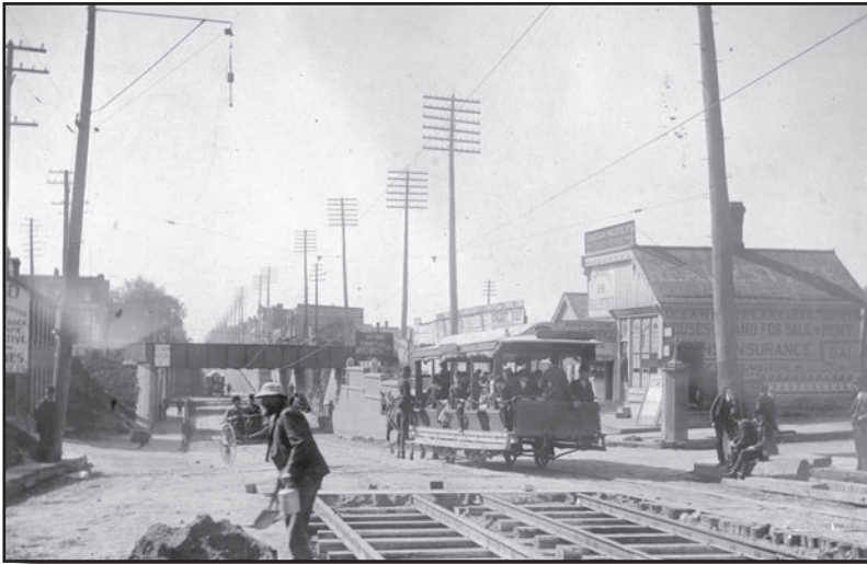
Making the grade -- work on the Queen St. W. subway, looking West. Fonds 200 Former City of Toronto fonds. -1834-1997, Series 376 City Engineer's Dept. photographs. - 1891-1911, File 1, Item 32b
