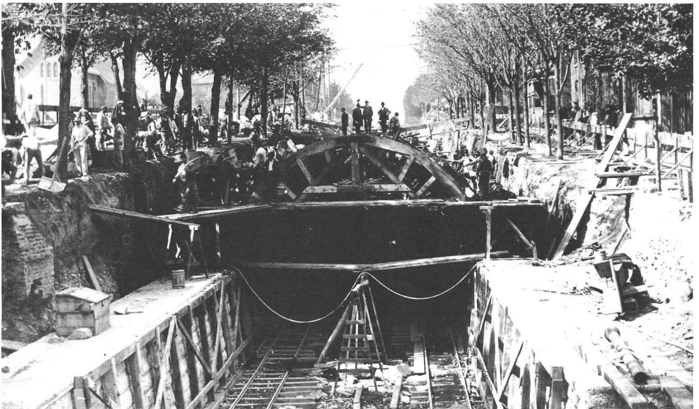
(Hamilton) Canadian railways usually crossed cities at grade level or through open cuts. The Toronto, Hamilton and Buffalo Railway built a tunnel in 1894 only where it passed through an elite neighbourhood. British cities insisted on high-standard work along railway rights-of-way. (photo: Hamilton Public Library)
