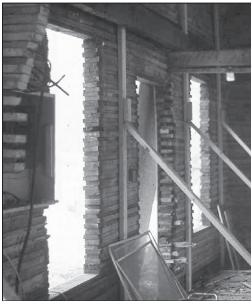
FIGURE 2. Short 'seconds' left over from the sawmill were nailed together in the plank-on-plank construction technique. Planks were offset in order to provide an uneven bonding surface for stucco and plaster. This is 7067 Pond Street during rebuilding in February 1985. (Author's photo)
