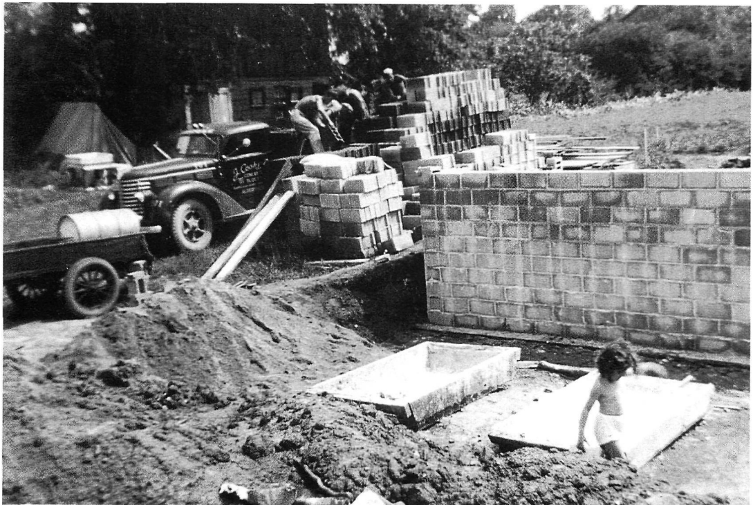
Figure 6: More blocks being delivered by the J. Cooke, Concrete and Blocks Company of Aldershot to complete the foundation, as Glenda Hall, their youngest daughter, wanders by the site, June
