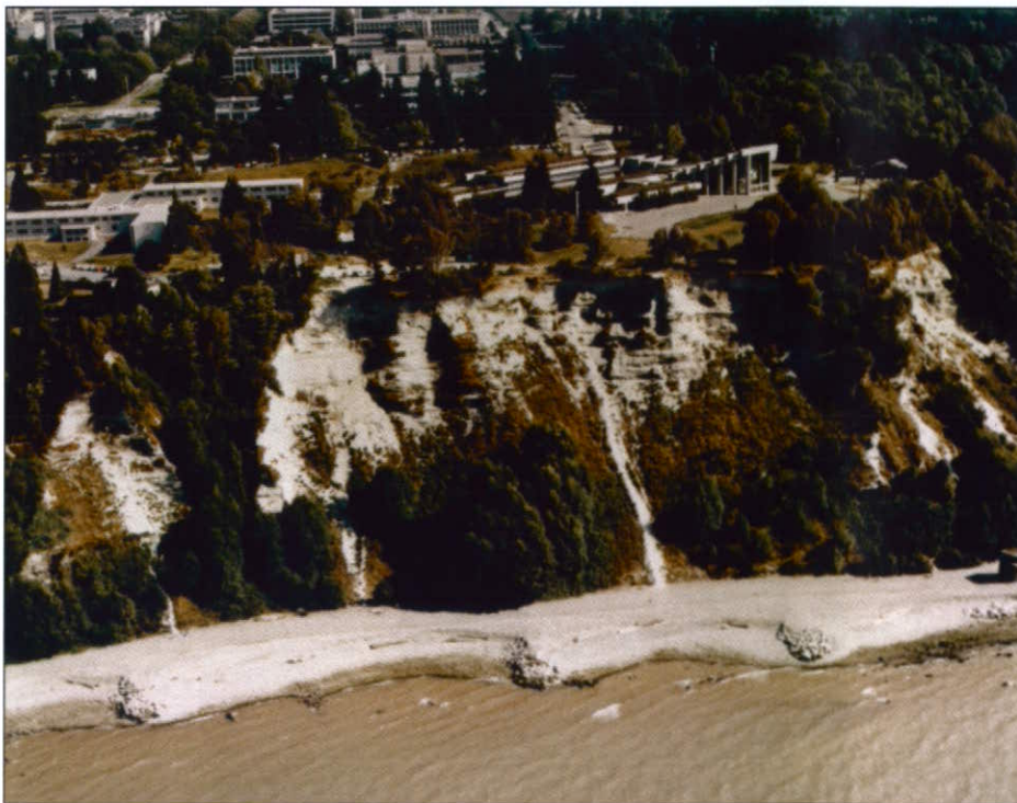
Figure 7 Eroding sea cliff at Point Grey, near Vancouver. The cliff is formed of loose sands and silts. It retreated at rates of up to 60 cm per year before 1982, when coarse gravel was placed at the shore to protect the base of the cliff from wave erosion (University of British Columbia, Campus Planning and Development).
