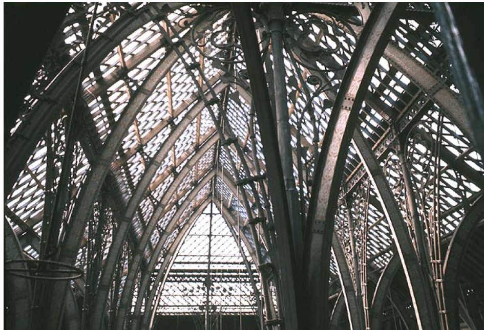
Figure 2: Oxford University Museum of Natural History, iron and glass roof. Photograph by George Landow, 1977, courtesy of the Victorian Web at http://www.victorianweb.org/art/architecture/oxford/19.html
